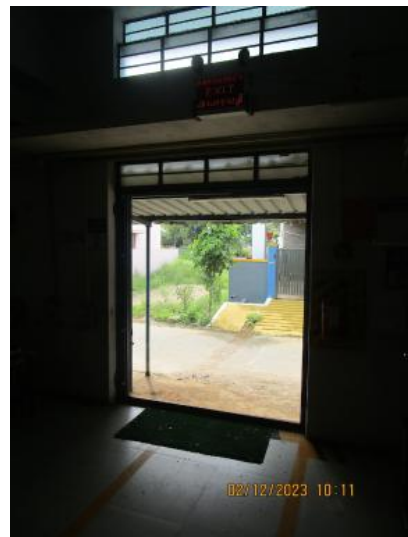
Emergency exit door.JPG
