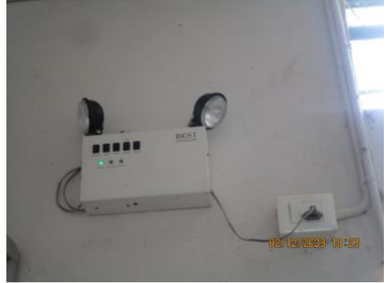
Emergency light system.JPG
