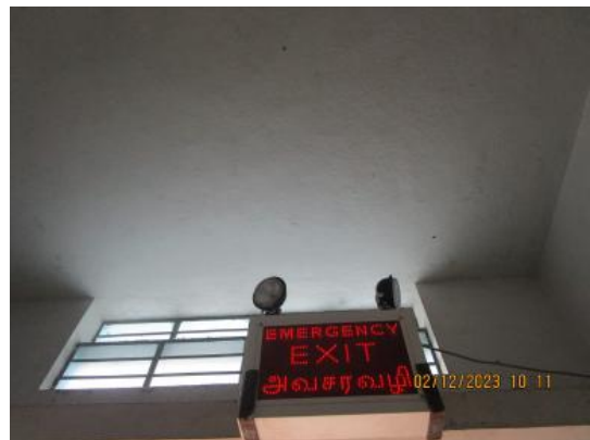
Emergency exit light .JPG
