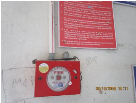
Emergency alarm call point.JPG
